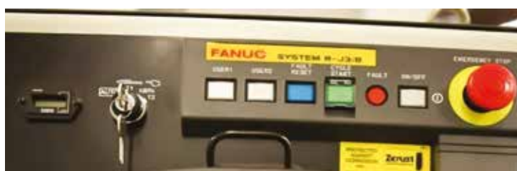
The control panel buttons of the Fanuc robot
