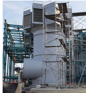
Cooling towers dia 6 m
