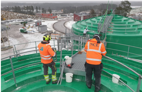
Tanks dia 15 m, 2120 m 3 /pc
